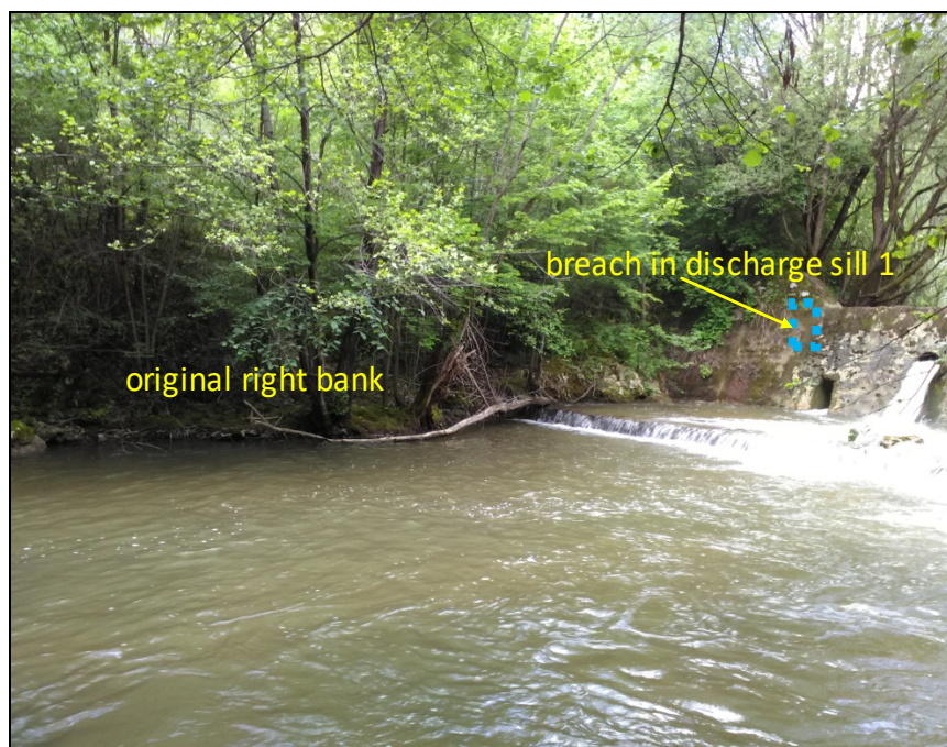
Figure 6: Downstream view of the breach.
