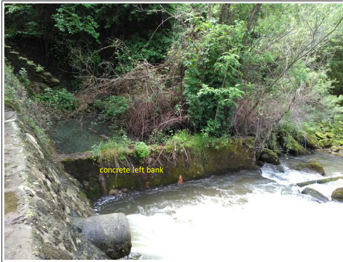
Figure 4: Concrete left bank of the Caraş River upstream of the discharge sill 1.
