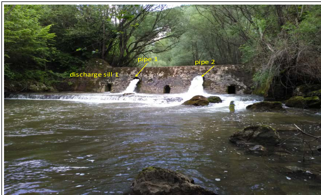
Figure 3: The first discharge sill threshold and the positioning of the two pipes.
